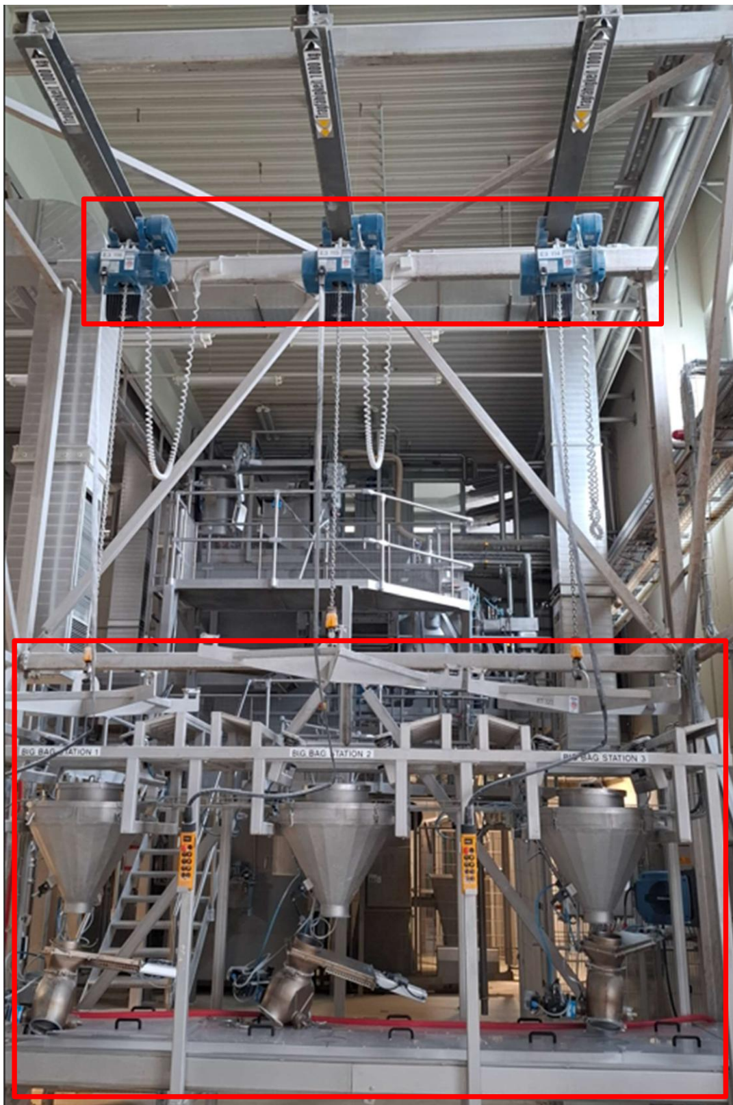
03. big bag station: Frame, chain lifts, bb hanging system, containers, slider, conveyor belt
