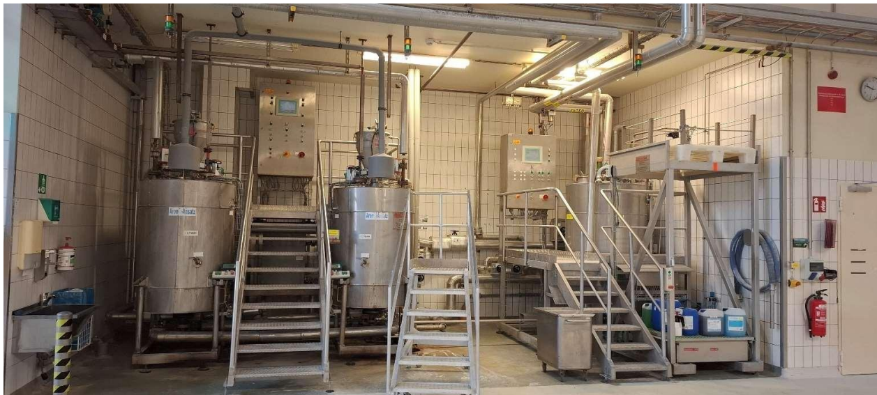
06. Liquid HCL, water and Oil Dosing
