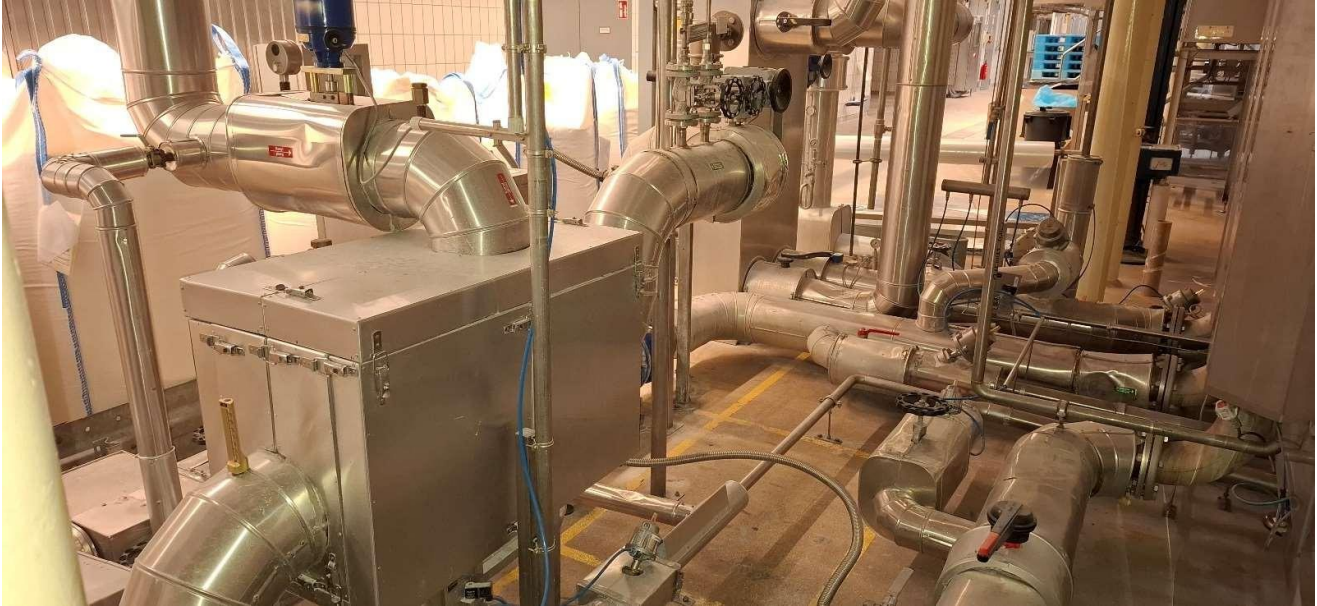
27. Heat exchanger for Pasteurizer 1
