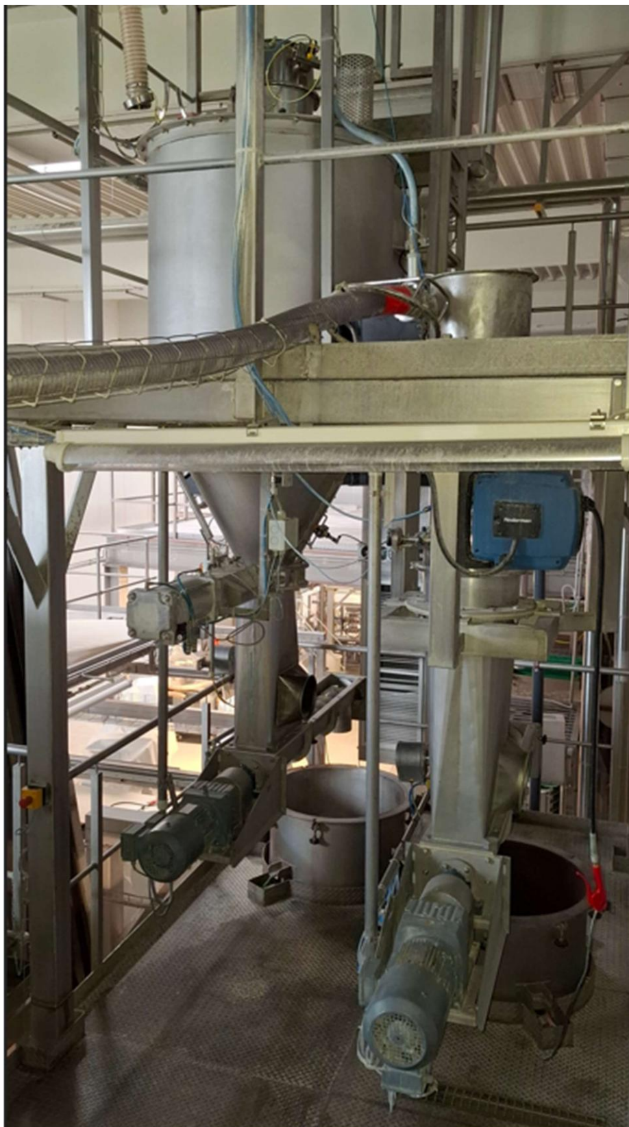
04. vakuum conveyors, component dosing, weighing container, platforms
