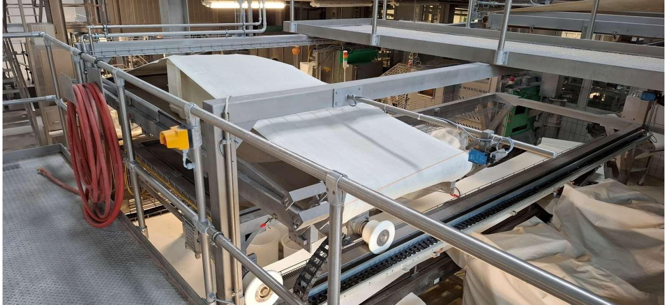
13. moveable conveyor belt
