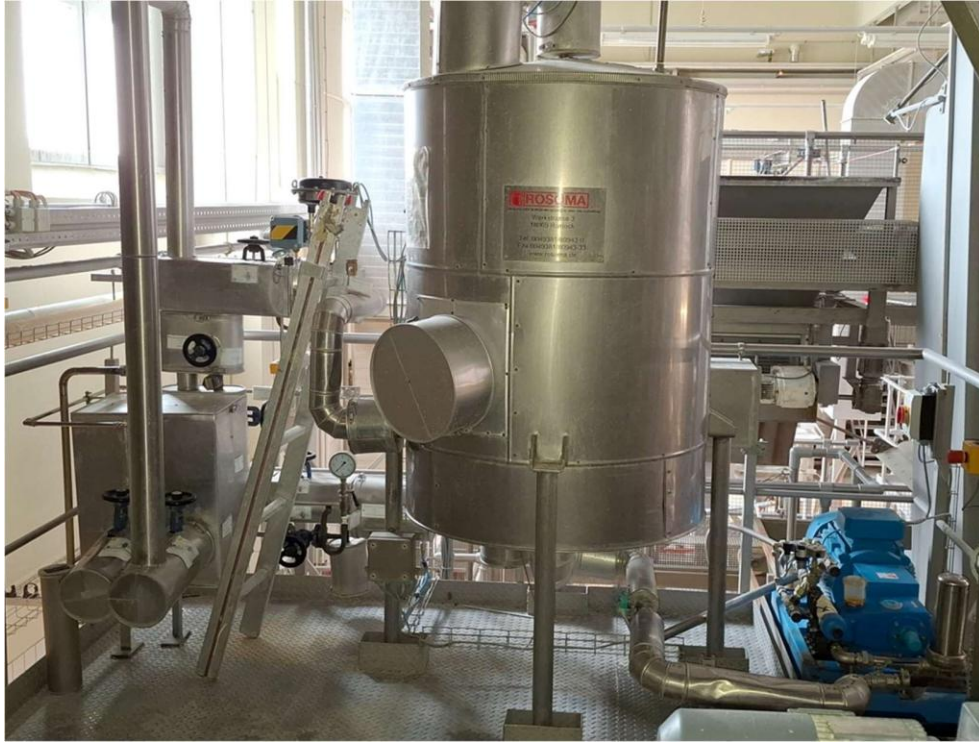
09. water preparation for cleaning station
