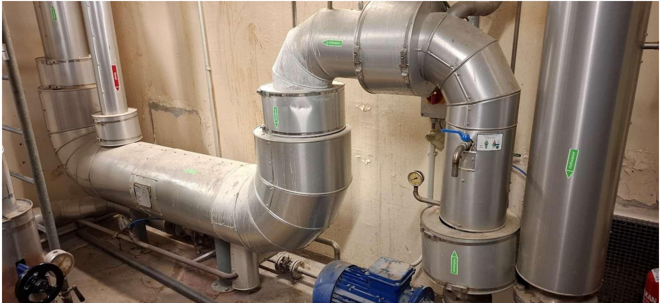
31. Heat exchanger for pasteurizer 2
