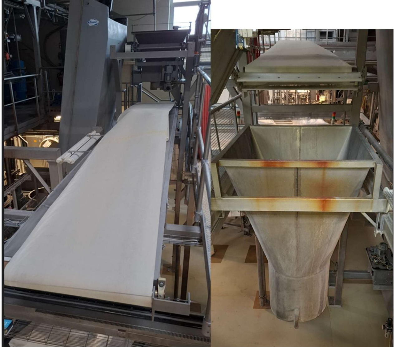
11. hopper with rollers inside, conveyor belt, hopper pipe
