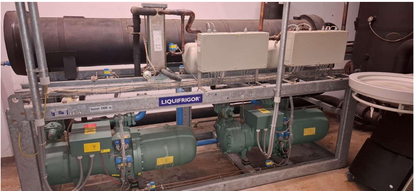
28. Cooling water system Liquifrigor for Pasteurizer 1
