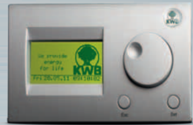
Boiler control unit
