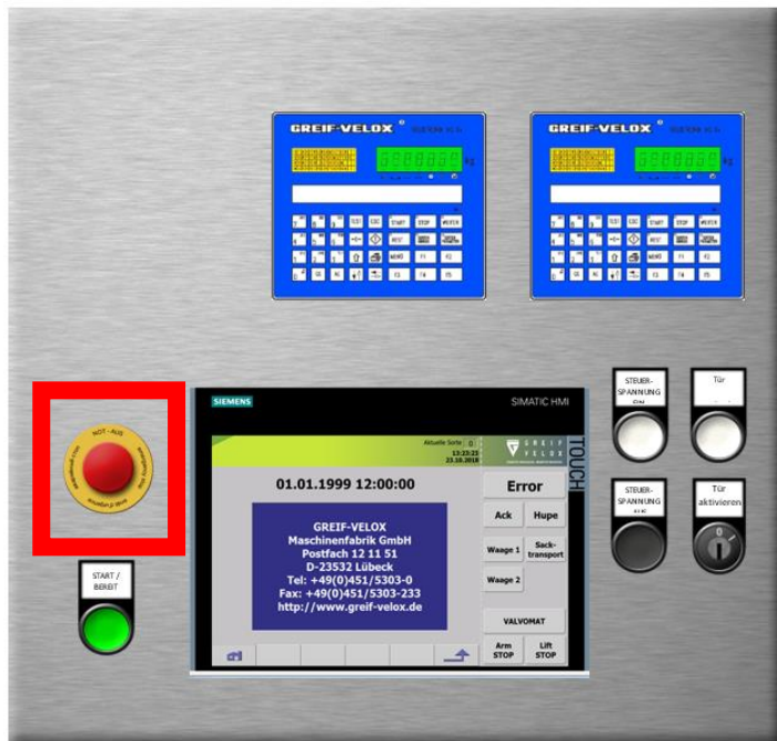
Figure 2 "Emergency Stop" on the control cabinet (1)
