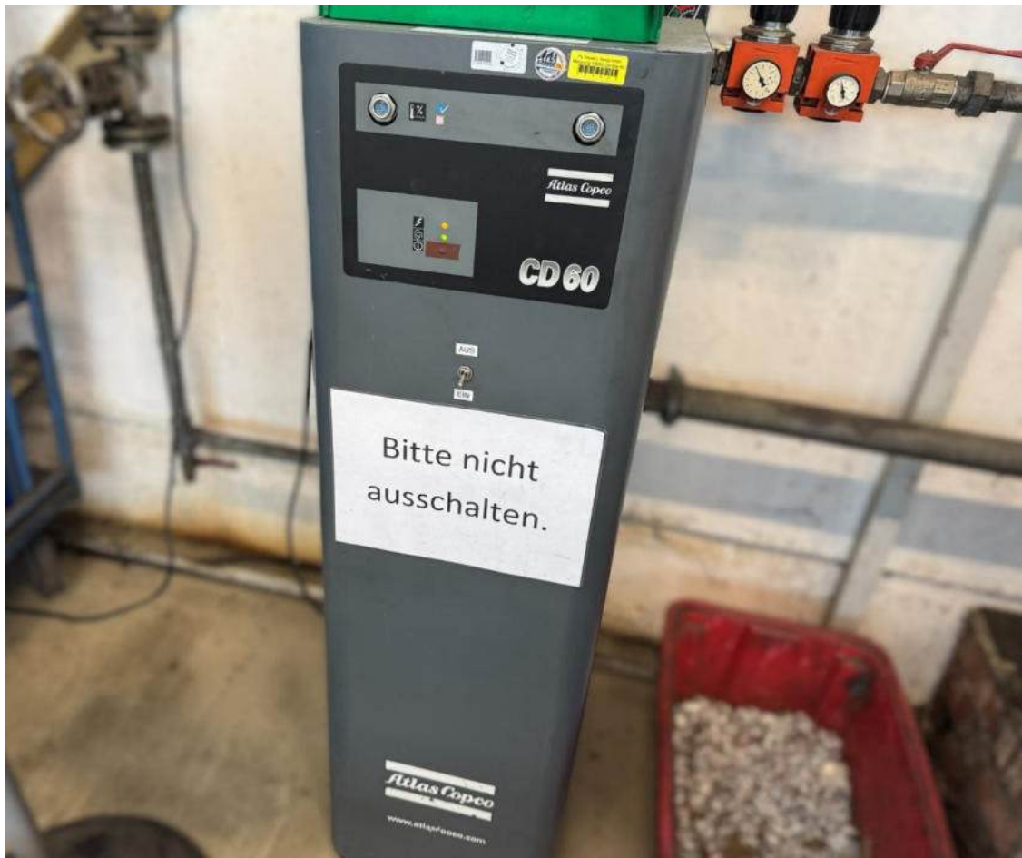
AIR DRYER ATLAS COPCO CD 60 - 2003
