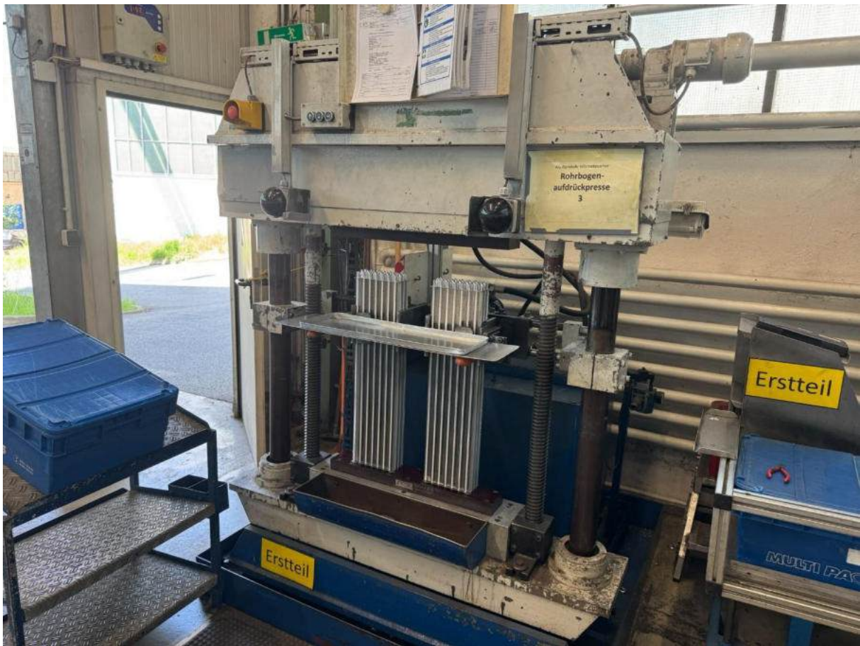
Pipe-Bend Pressing Machine 3
