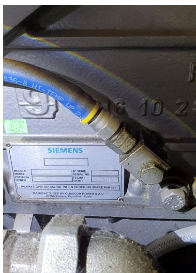
Motor - Siemens / Guascor
