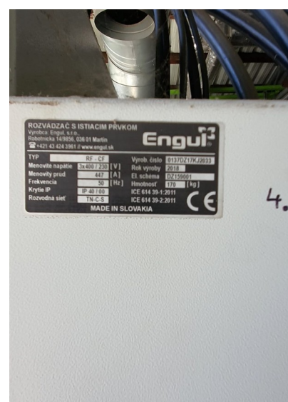
Control cabinet - Engul
