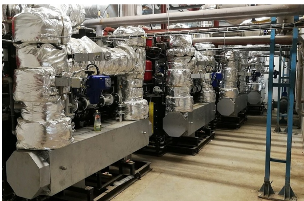
Heat recovery and piping equipment
