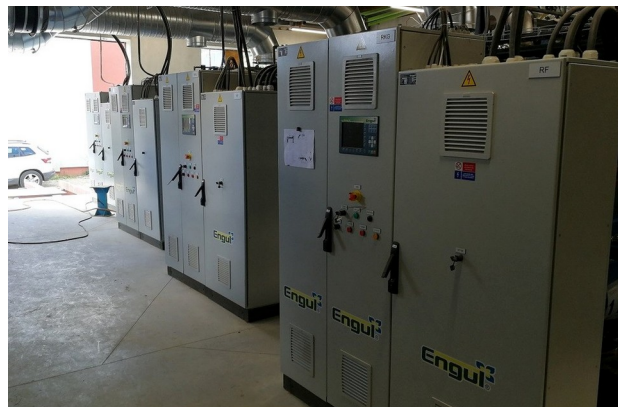
Control cabinet lineup / control system
