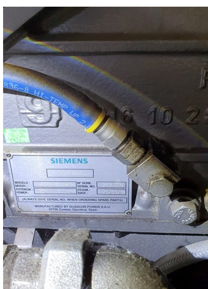
Engine - Siemens / Guascor
