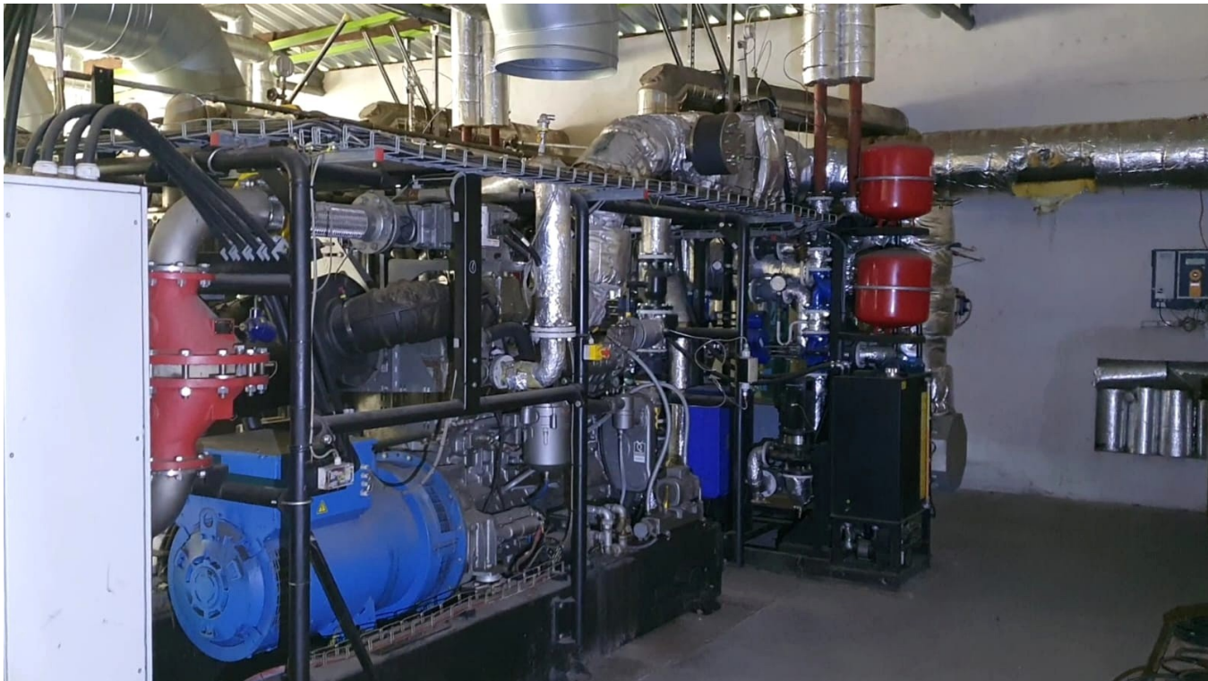
Figure: existing open-skid CHP units in the engine room
