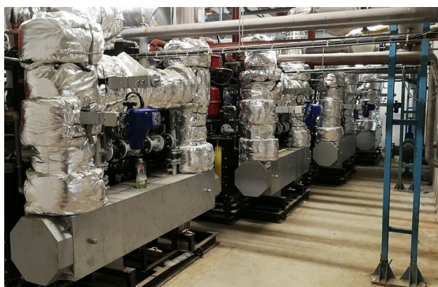
Heat recovery / piping
