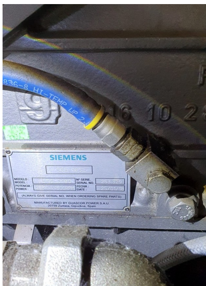
Motor - Siemens / Guascor
