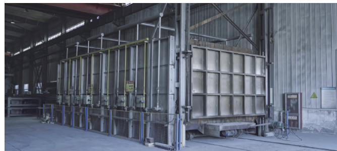
Gas truck style thermal treatment furnace
