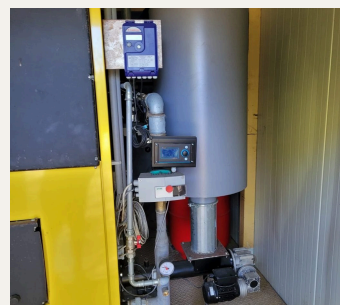
Cyclone, flue fan & feed
