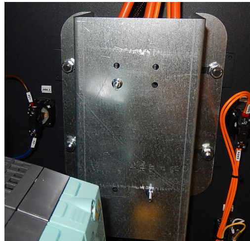
Figure 1-7: Printer Main AC Breaker cover
