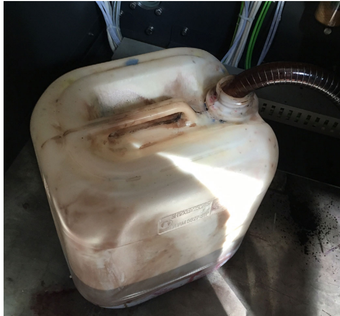
Figure 1-23: Waste line and Waste Tank
