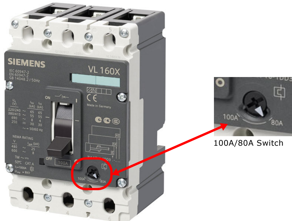
Figure 1-6: Printer Main AC Breaker, with 100A/80A Switch highlighted
