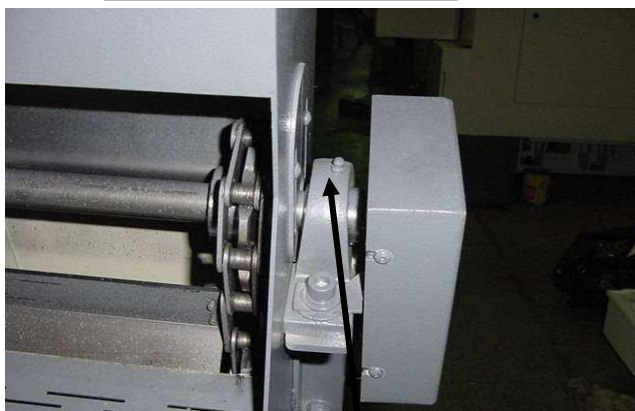
Chip conveyor bearing housing #2
