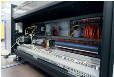
CE and UL certified electrical installation.
