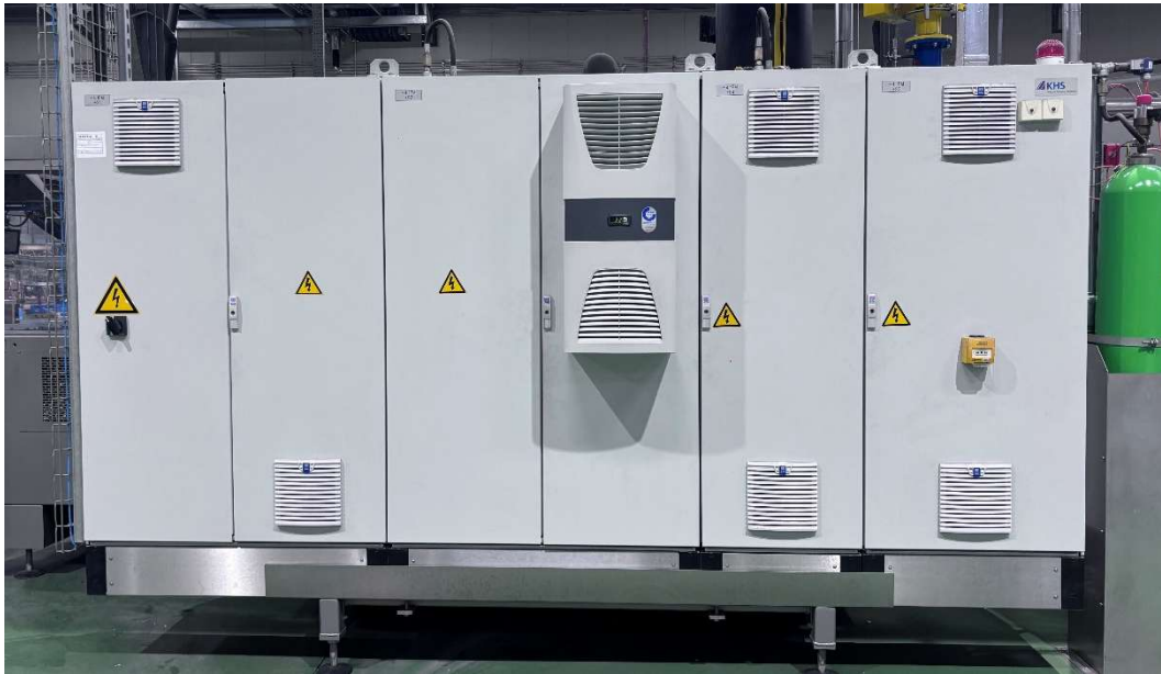
Electrical cabinet: 4000mm x 1200mm
