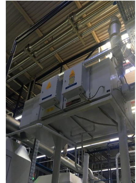
Peripherie Absaugung ( extraction system )
