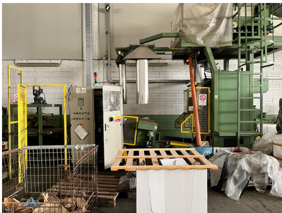
1 — CTS 80 bagging machine and control panel
