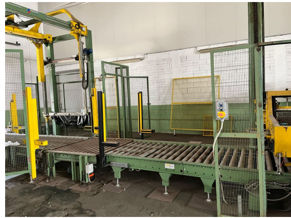
4 — Roller conveyor and pallet output
