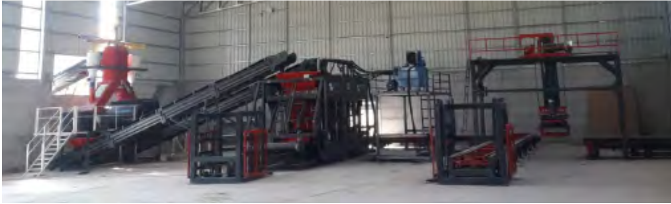
Filistin - ZIM 1230 U Tipi Beton Parke ve Blok Üretim Tesisi Palestine - ZIM 1230 U Type Concrete Pavers and Block Production Facility
