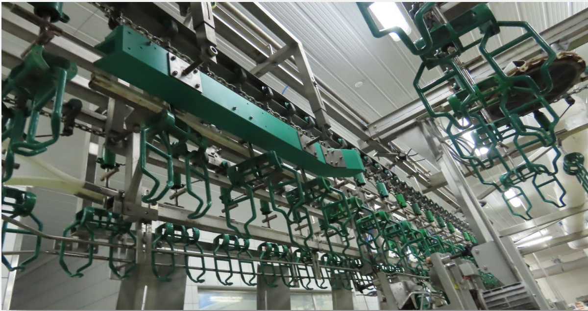
Picture 21: Support structure: OHC, drives, hangers
