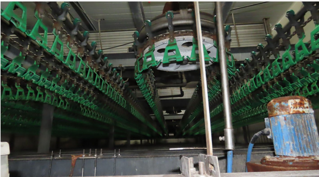
Picture 5: Tunnel (on the upper floor) with evaporators
