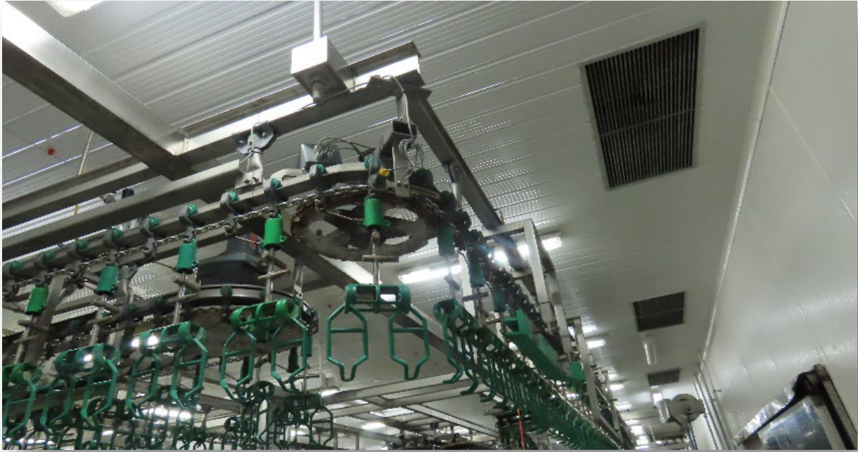
Picture 20: Support structure: OHC, drives, hangers
