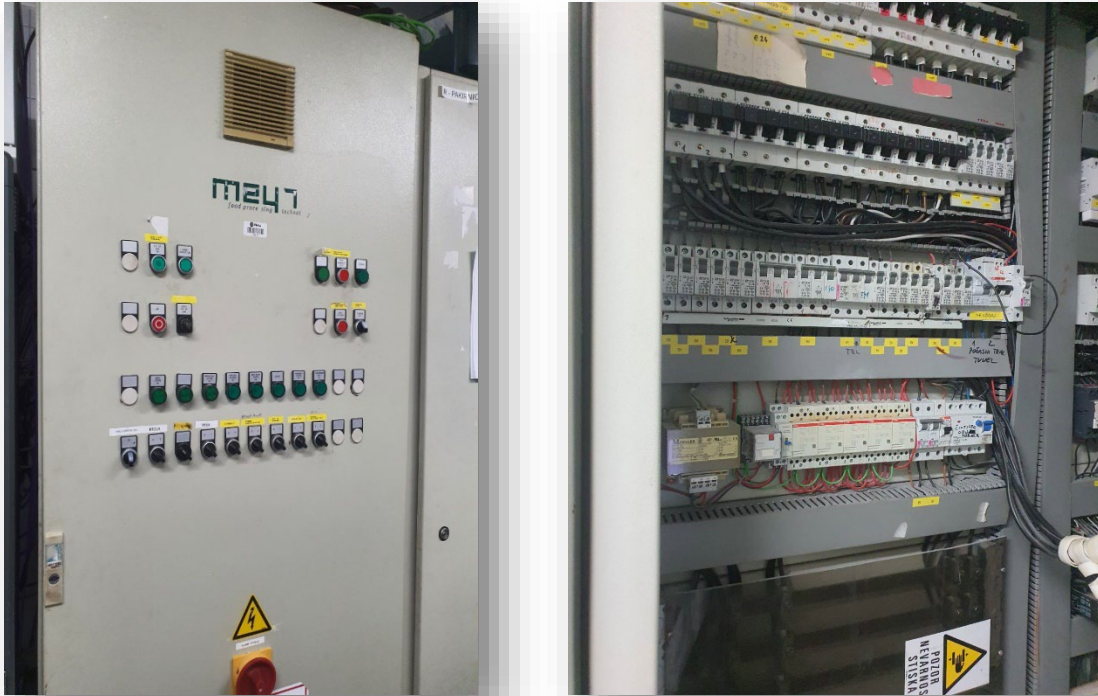
Picture 15: Electric cabinets (section)
