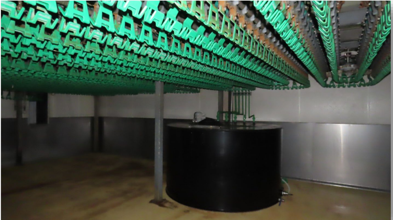
Picture 4: Tunnel (on the lower level) with tanks for liquid ice
