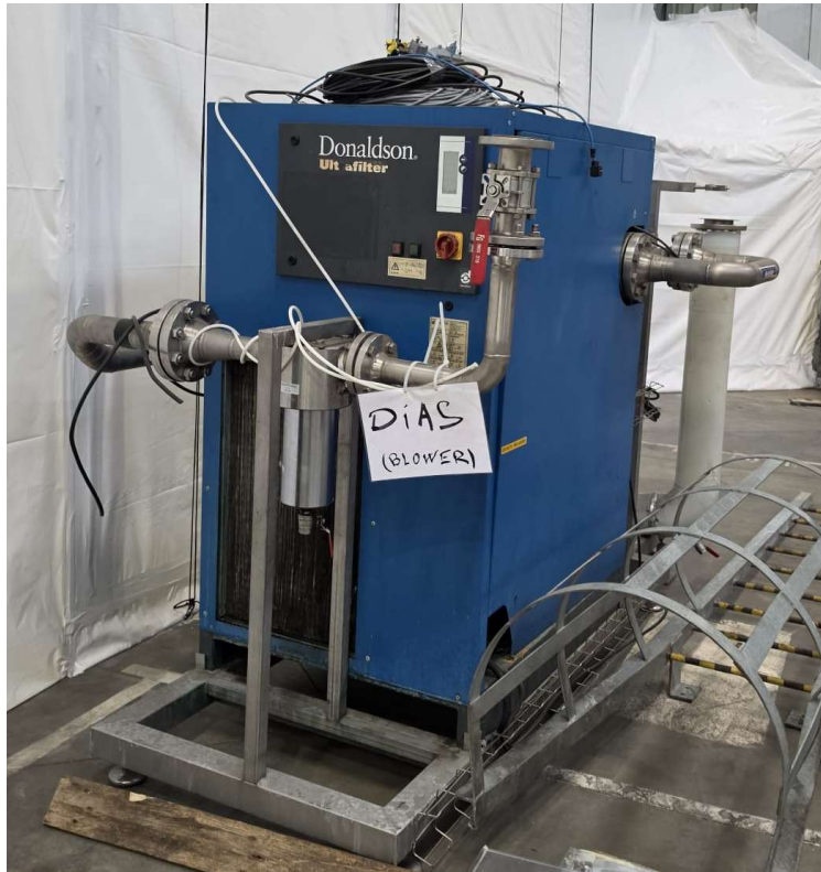
compressed air dryer: 1800mm x 1000mm
