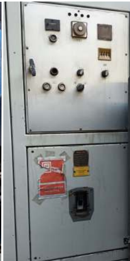
Device Cabinet - Commande
