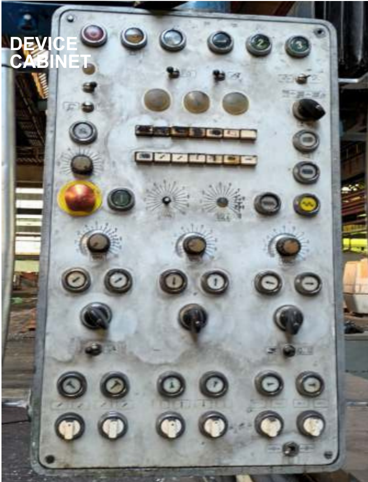
Main Control Panel
