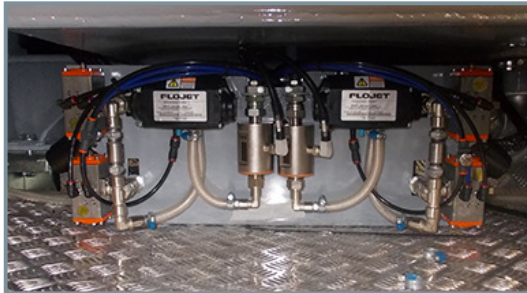
Liquid additive dispensers with flowmeters
