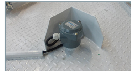
Level sensor on the binder silos with alarm siren
