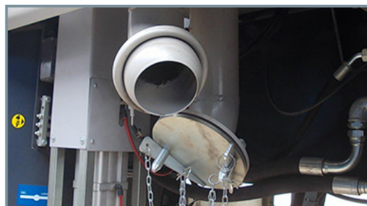
Pipes for pneumatic refilling of the binder silos
