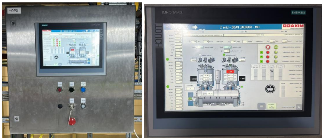
Left: HMI hot mixer Right: main page hot mixer (from main plant with two Hot mixer)
