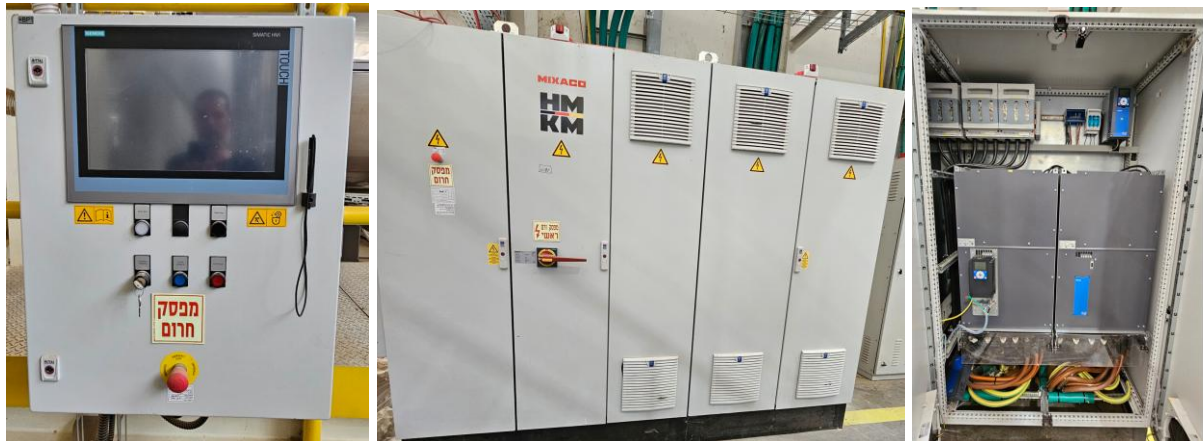
Left: HMI for cooling mixer Mid: main electric cabinet Right: VFD Vacon
