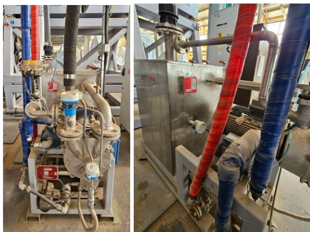
Left: vacuum pump Right: vaccum pump tank
