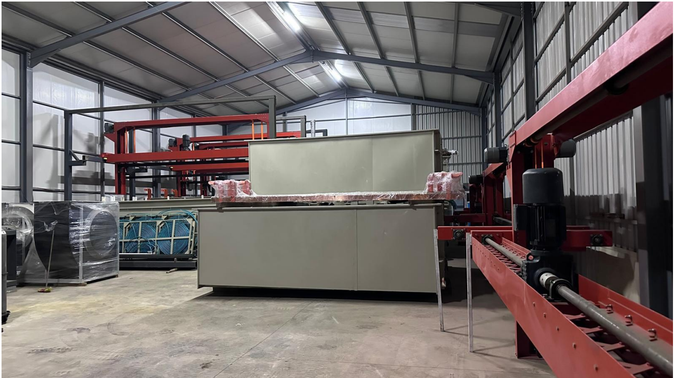
Refurbished line and tank assembly
