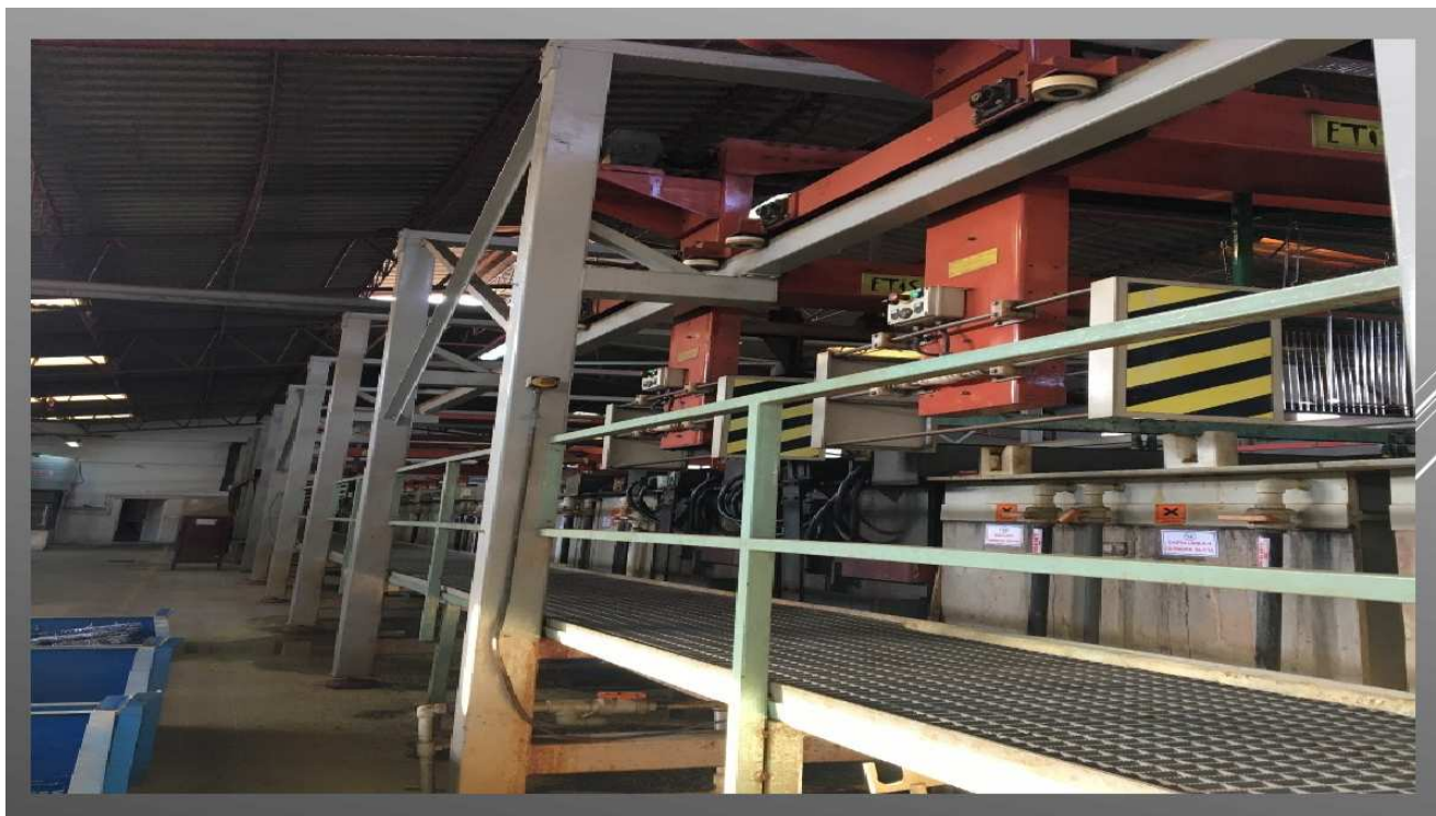
Transport system alongside the process tanks (historical source slide 9)
