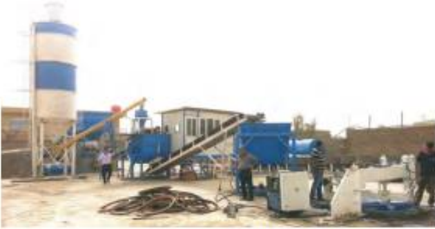
Irak - ZIM Y 1200 Beton Boru Üretim Tesisi Iraq - ZIM Y 1200 Concrete Pipe Production Facility
