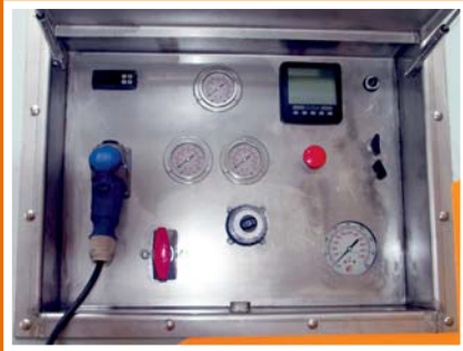
Shielded Control Panel.
