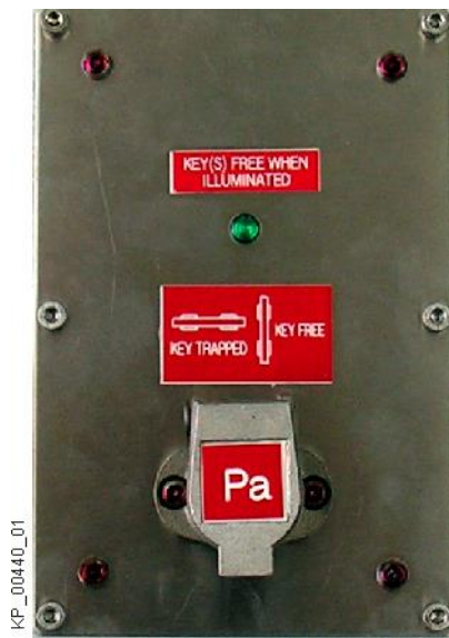
Fig. 2: Lock on the switch cabinet
