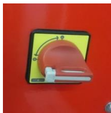
Pic. 7 Main power switch
