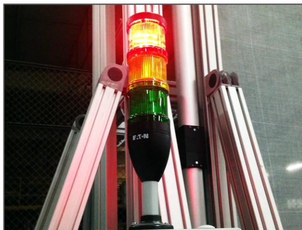
Figure 23: Light tower on the electrical cabinet
