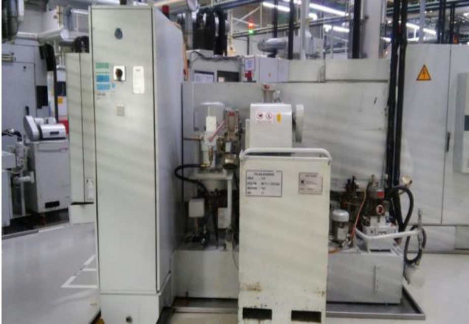
Periph. Rückpumpstat. ( return pumping station )
