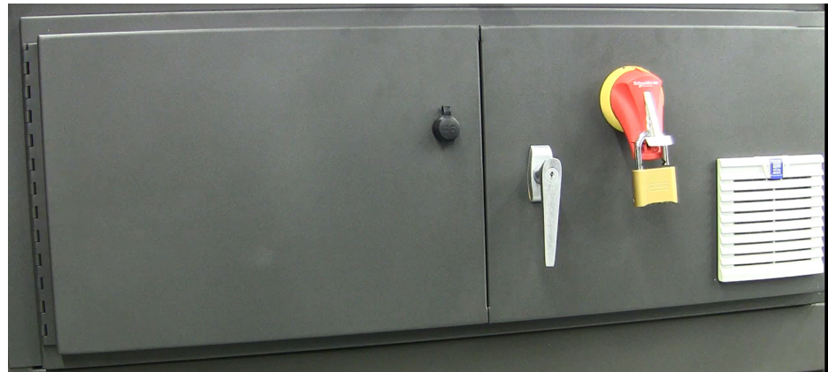
Figure 2-3 Electrical Box cover and handle
