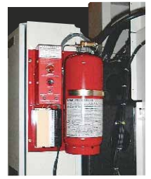
Automatic fire extinguisher (Note)
