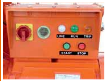
Die cast electrical box with main switch, overload relay & hour meter.
