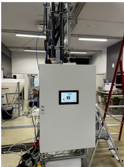
Control cabinet in service — touchscreen and a neatly equipped Rittal enclosure.
