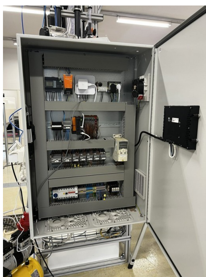
Control cabinet — B&R PLC, I/O and power supplies
